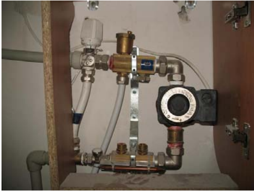
The heating system was remade and upgraded: now there is the heat-insulated floor and a dryer in the house.
